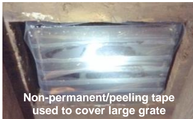
Figure 5. Inappropriate basement air sealing
